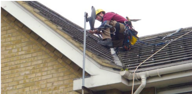
191m of black Flex-Track was chosen by Igrox to blend in with the grey roof tiles.
