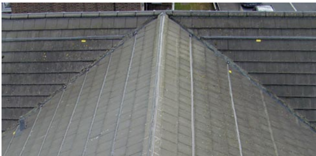
Quick Tap Jumpers were used at each end to connect the multiple rows. Warning Signs were glued in place on the roof tiles.
