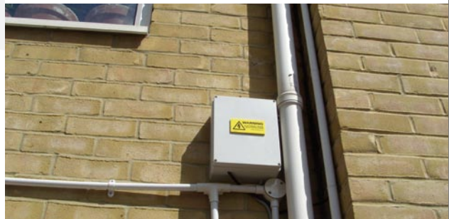
The Energiser was sited in a waterproof external box. This allows isolation of the energiser by maintenance personnel without disturbing the tenants.
